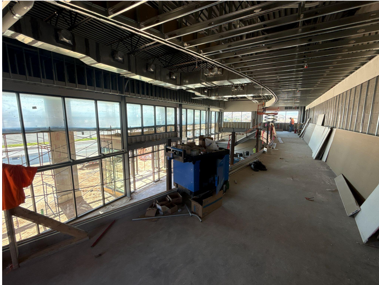
Interior view of the Dimon Legacy Theatre under construction, St. George, Utah, 2026.
