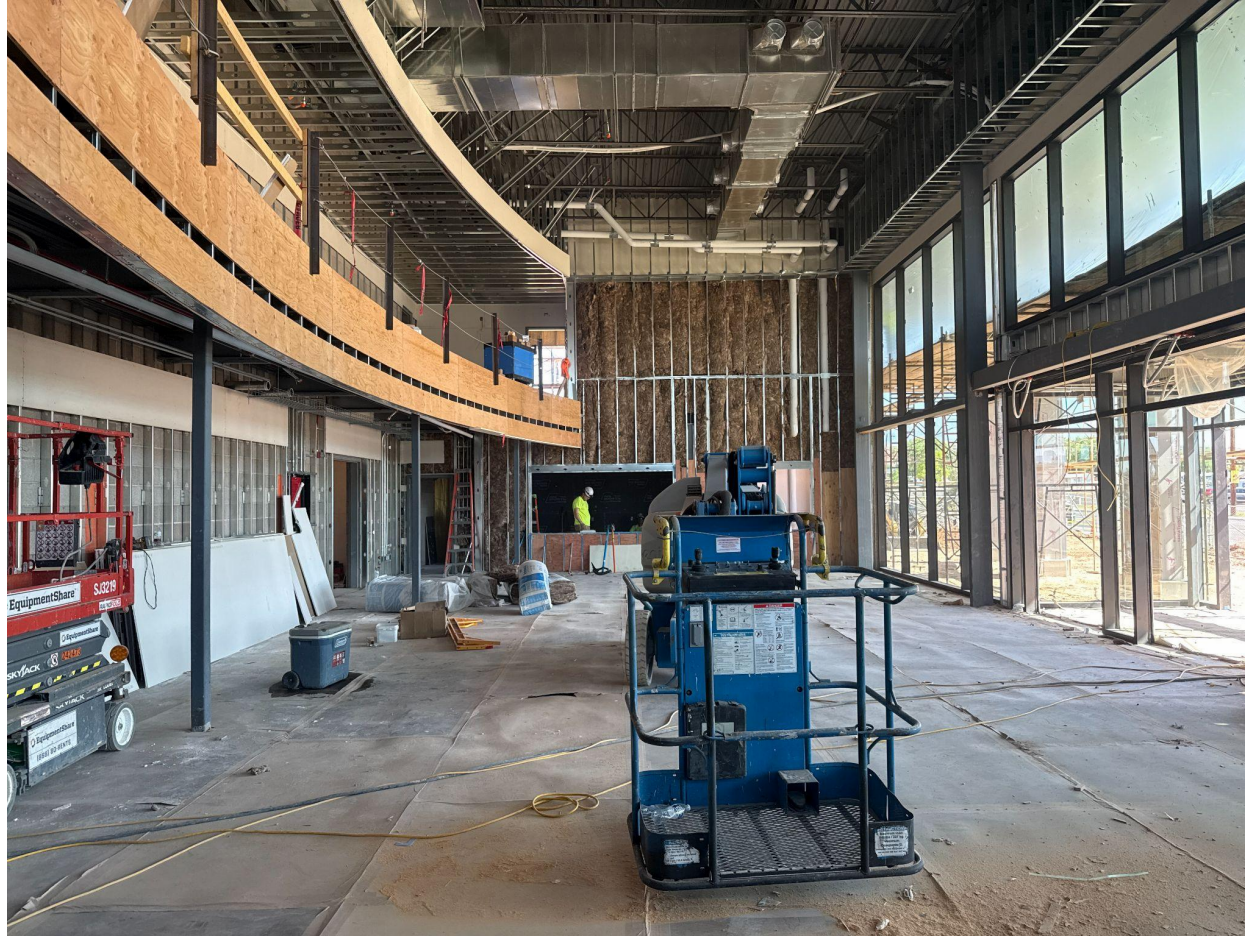
Interior view of the Dimon Legacy Theatre under construction, St. George, Utah, 2026.
