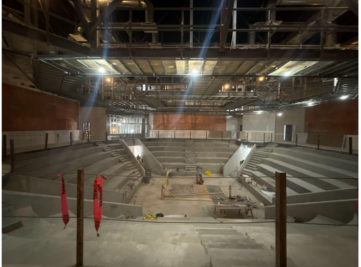
Interior view of the Dimon Legacy Theatre under construction, St. George, Utah, 2026.
